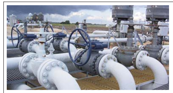
Salt Dome Brine & Gas Pumping Station
