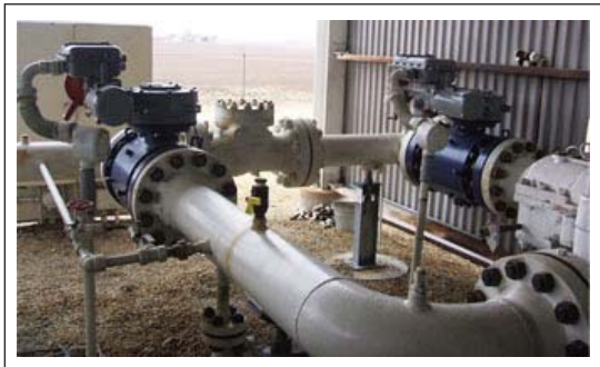
Crude Oil Pumping Station Pig Launcher/Receiver
